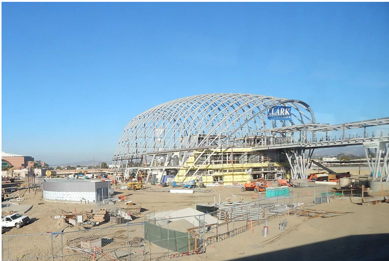
Recent construction underway in Anaheim for the Anaheim Regional Transportation Intermodal Center (ARTIC) scheduled to open at the end of this year. Photo by Noel T. Braymer
