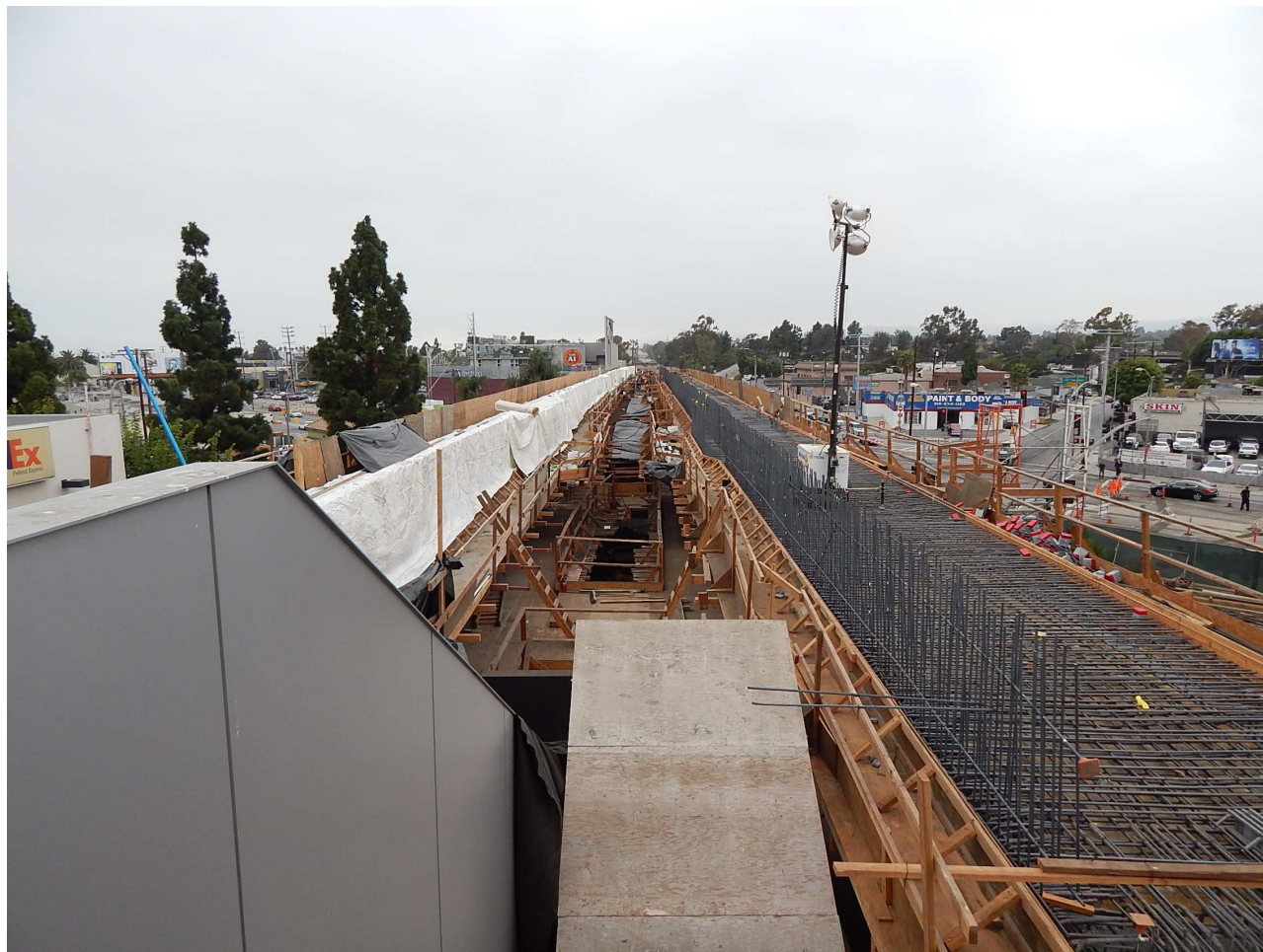
The view from the Culver City Expo Station at the viaduct over Venice Blvd under construction. Photo by Noel T. Braymer
